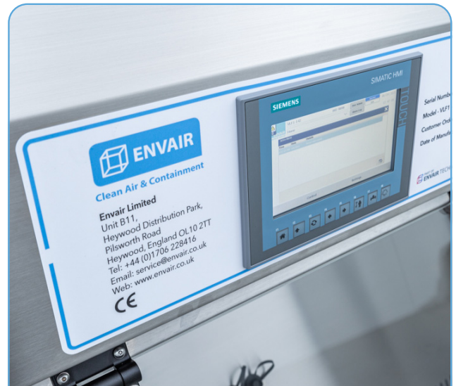
Siemens PLC control system
